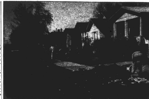
STREET IMPROVEMENT and drainage project underway along Myrtle avenue, being carried out with state motor fuel tax funds. Similar improvement programs also are slated for Sheridan and Jerden avenues in East Granite.
